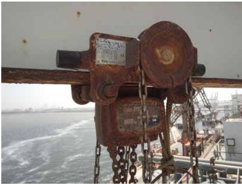
Corroded Yalelift with integrated trolley – still functional after 9 years in use
